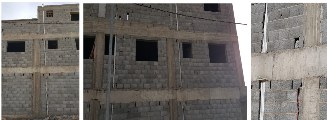
Fig. 1. RC floor beams with vertical pipe openings in the shear zone.
